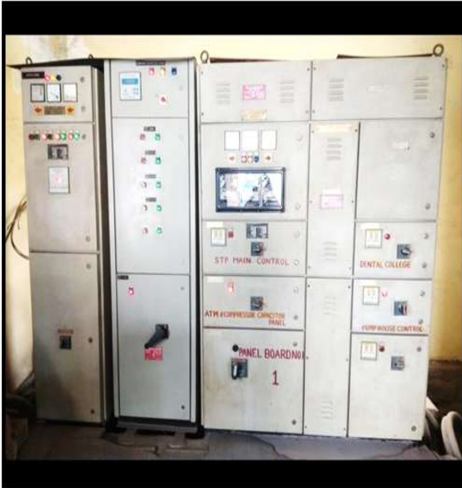
Control panel for the distribution and maintenance of water bodies in the campus.
