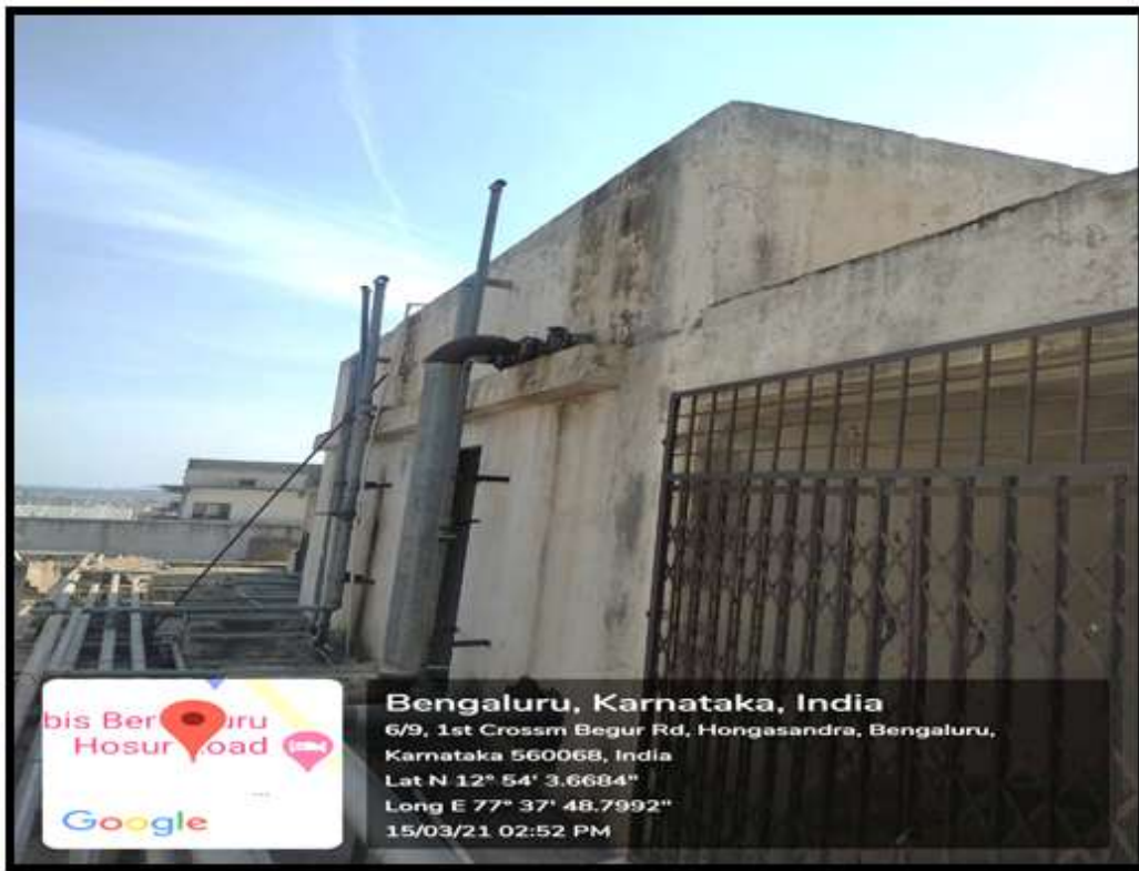
Overhead tank in the Girls hostel
